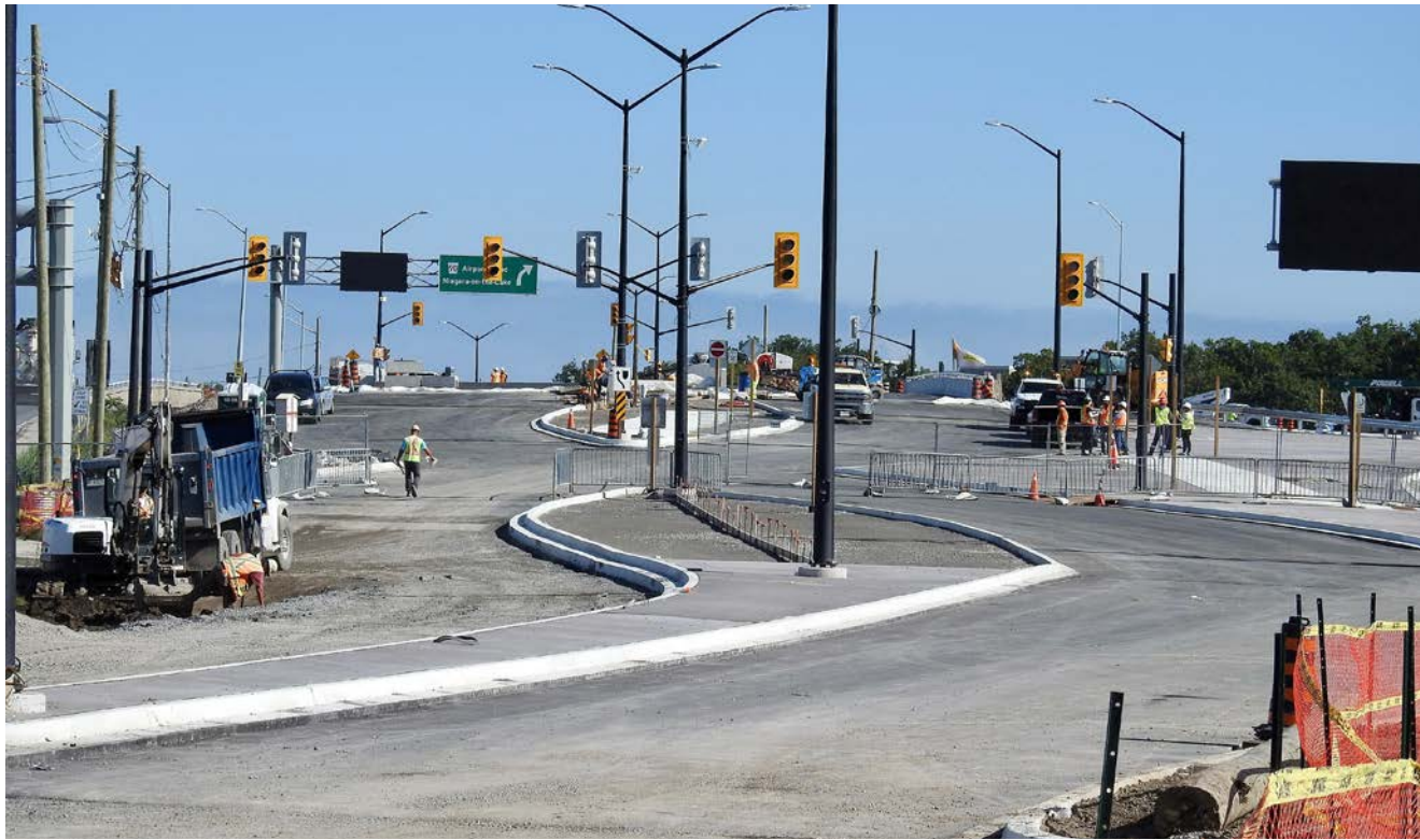
Construction workers continue to put the finishing touches on the QEW/Glendale Avenue diverging diamond interchange, with an opening planned for Monday, Sept. 26. STEVE HARDAKER
