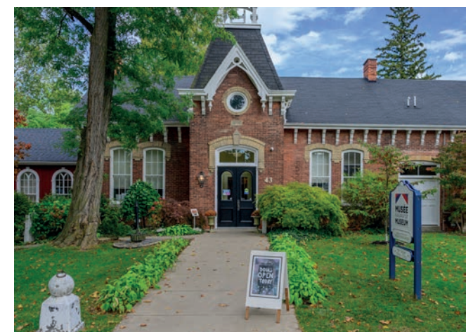
The NOTL Museum remains open during regular hours as construction on the expansion takes place next door.
