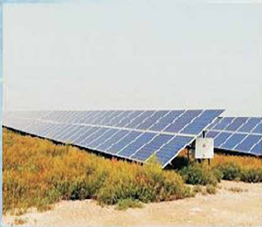
CASE6,5MWPOLYSOLARPANEL230W,INSTALLED INFIRENZA,ITALYIN2010COOPERATEWITH OVERIASOLARS.R.L
