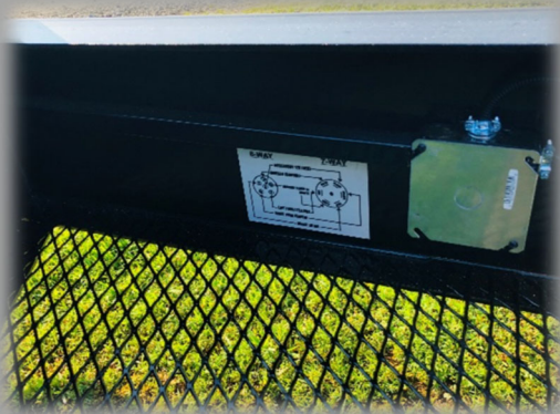
SEALED WIRING & LED LIGHTS
