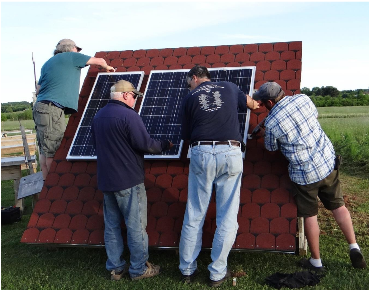
Figure 14 Panels going on – room for 2 ½ more as our need grows
