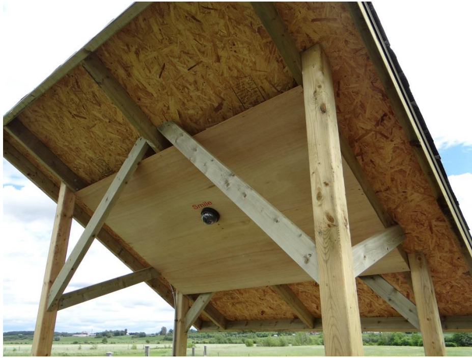
Figure 18 Bracing Added to Support Roof
