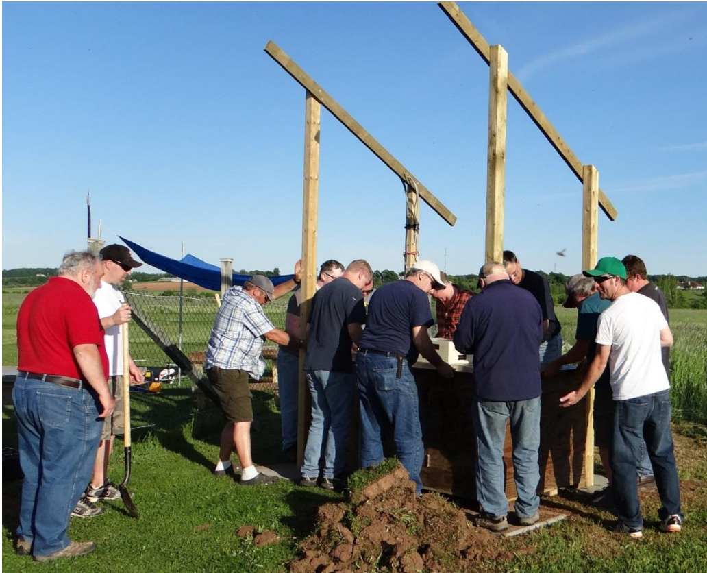
Figure 12 Aligning with solar south, 22 degrees west of magnetic south in Nova Scotia
