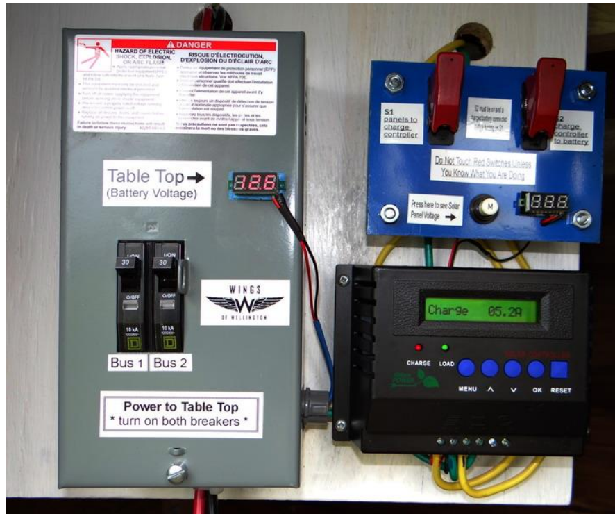
Figure 6 Panel – Green power 28 amp controller and two 30 amp circuits to the table through Square D breakers
