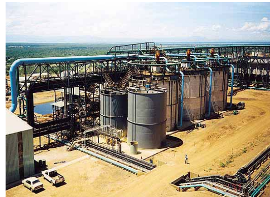
Fig. 9 Aerated stirred tank bioleach plant. Courtesy of Kasese Cobalt Company, Uganda.
