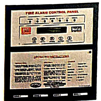
FIRE ALARM PANEL
