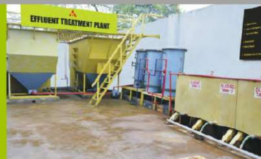
Effluent Treatment Plant
