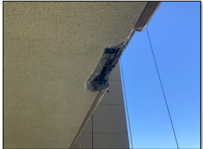
FIGURE 5 - Overall view of concrete removed around corroded rebar treated with corrosion inhibitor.
