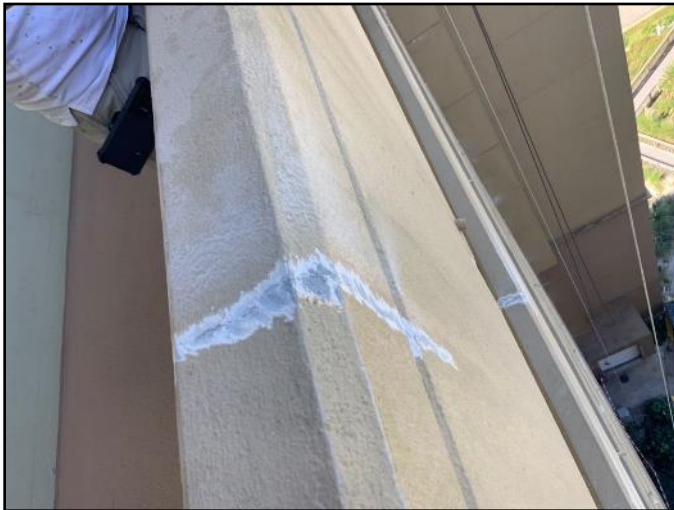
FIGURE 4 - Close-up view of finish material removed around concrete crack prior to routing and sealing.
