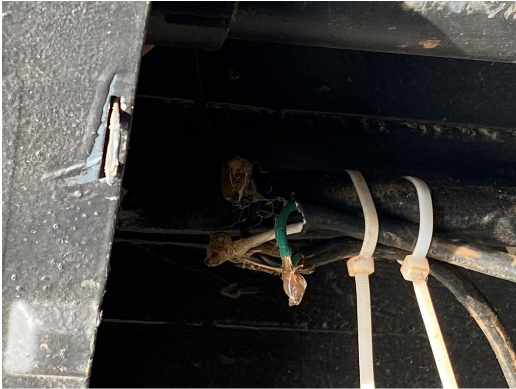
Electrical Code Photo 32
