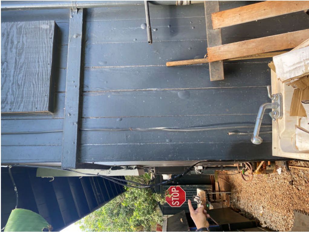
Electrical Code Photo 35
