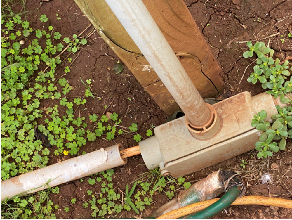
Electrical Code Photo 39
