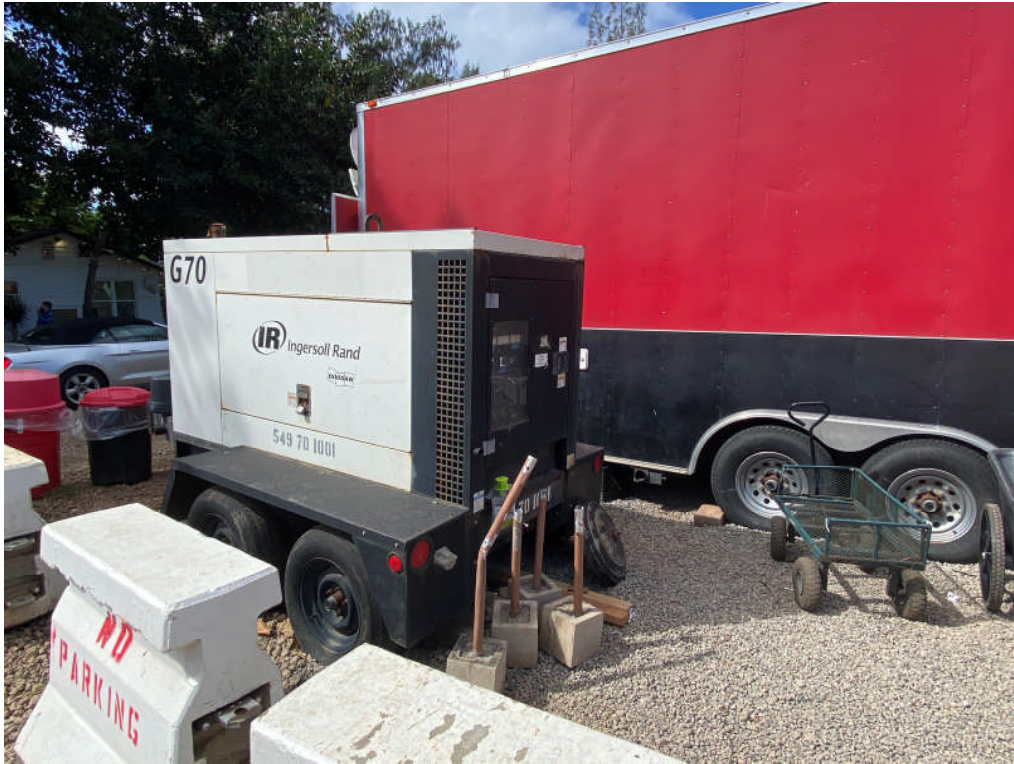
Electrical Code Photo 19
