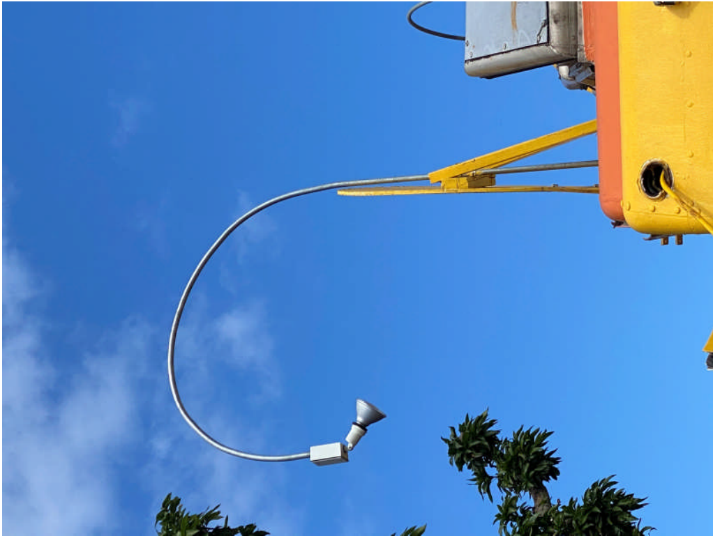
Electrical Code Photo 36
