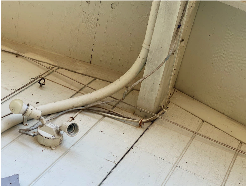
Electrical Code Photo 3
