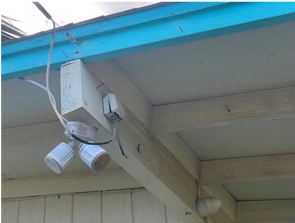
Electrical Code Photo 4
