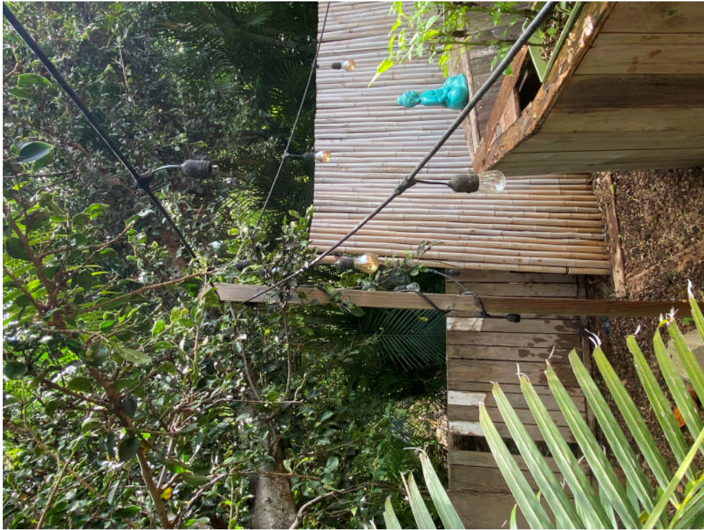
Electrical Code Photo 43
