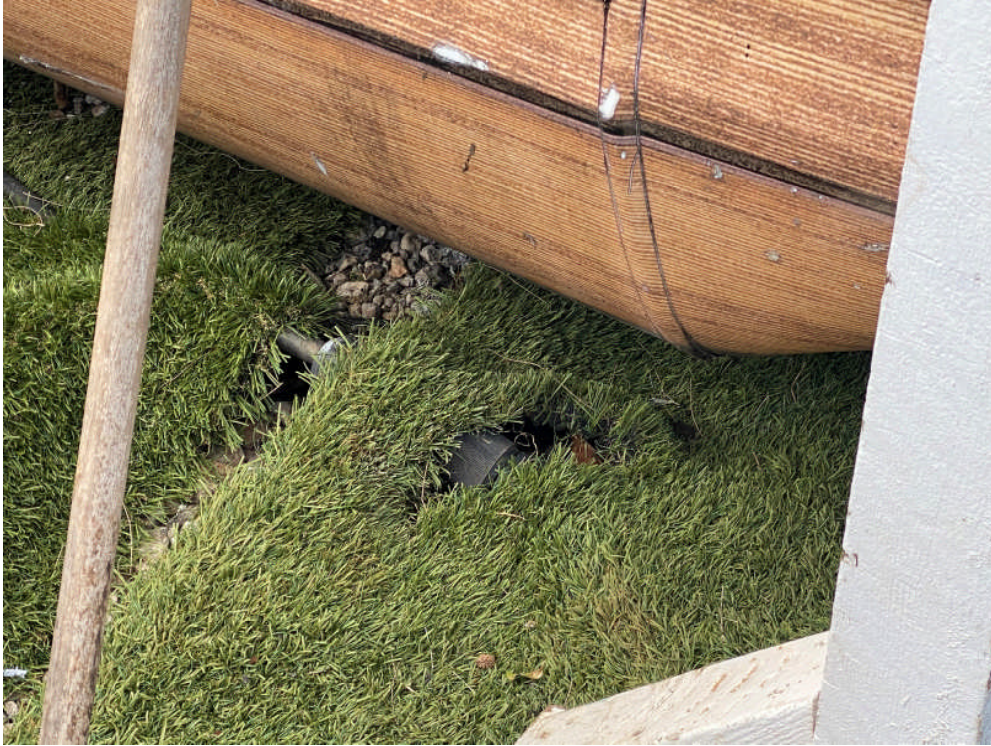
Electrical Code Photo 11
