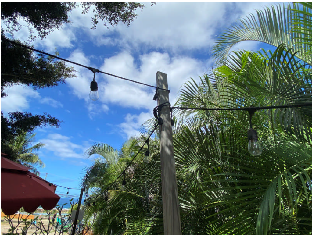
Electrical Code Photo 44
