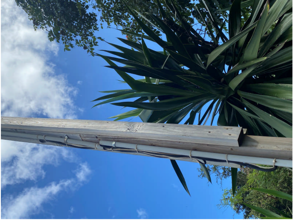
Electrical Code Photo 40
