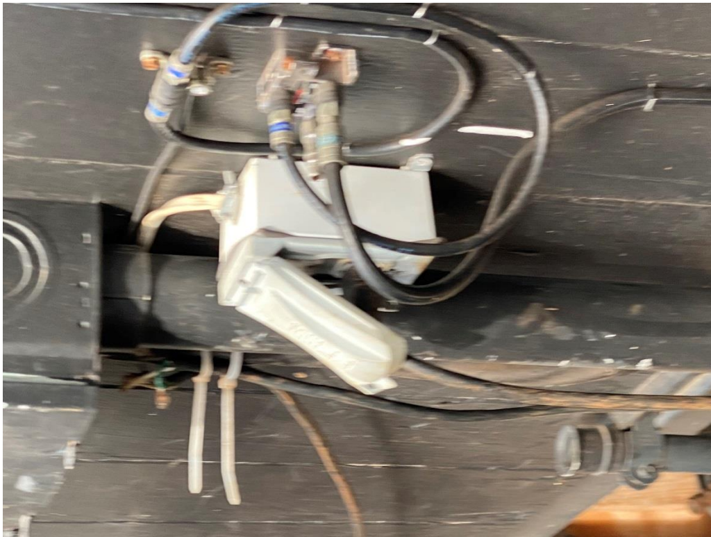
Electrical Code Photo 30
