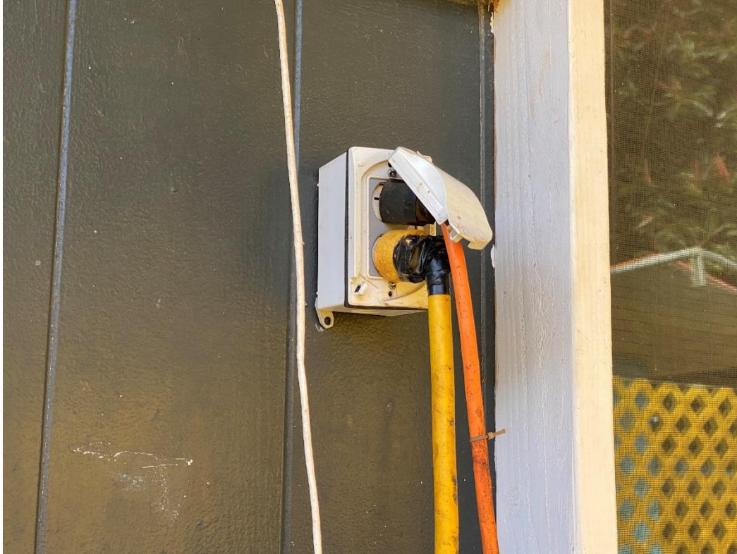
Electrical Code Photo 28
