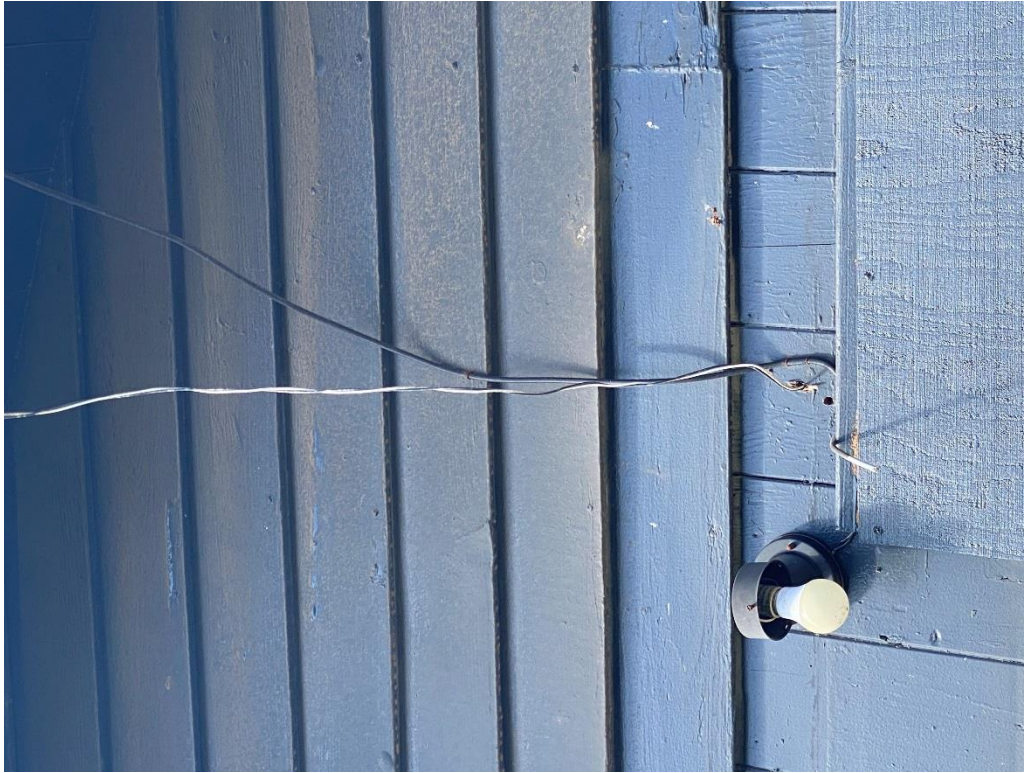
Electrical Code Photo 29
