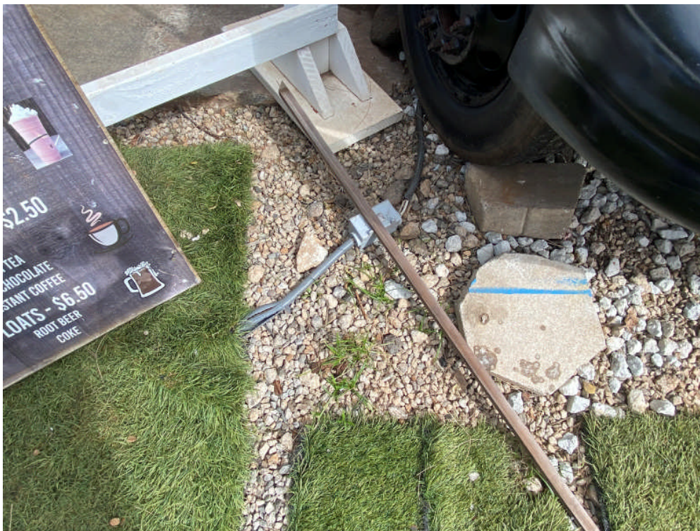
Electrical Code Photo 18
