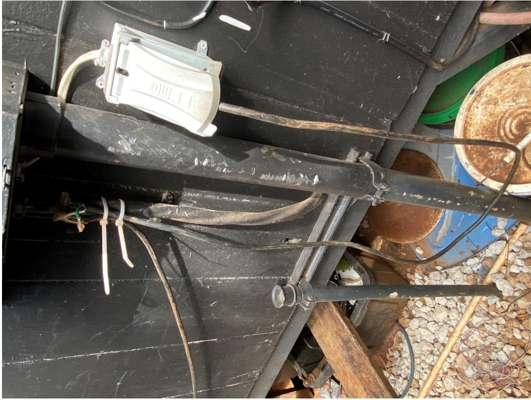
Electrical Code Photo 31
