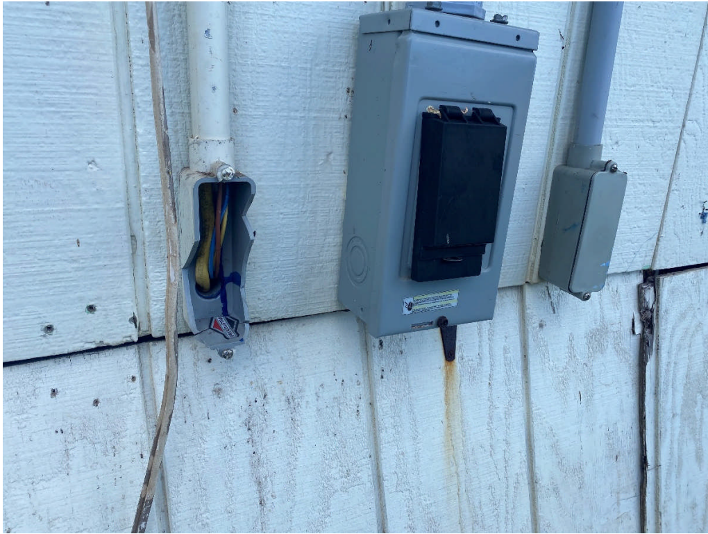
Electrical Code Photo 1
