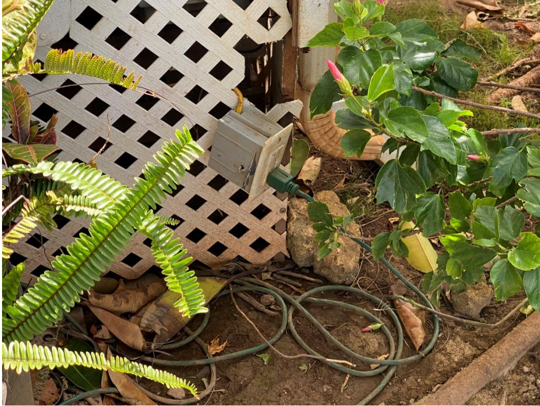
Electrical Code Photo 21
