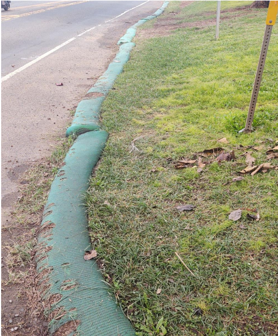
Pic 1; BMPs need to be addressed before start of grading/paving.
