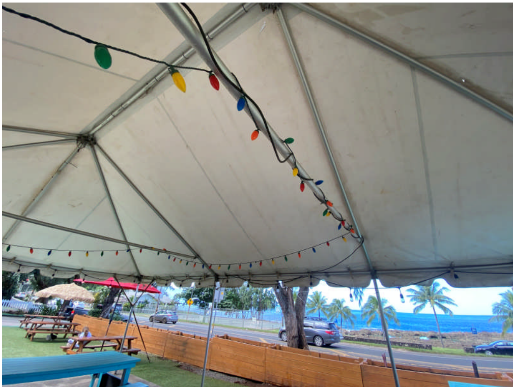
Electrical Code Photo 14
