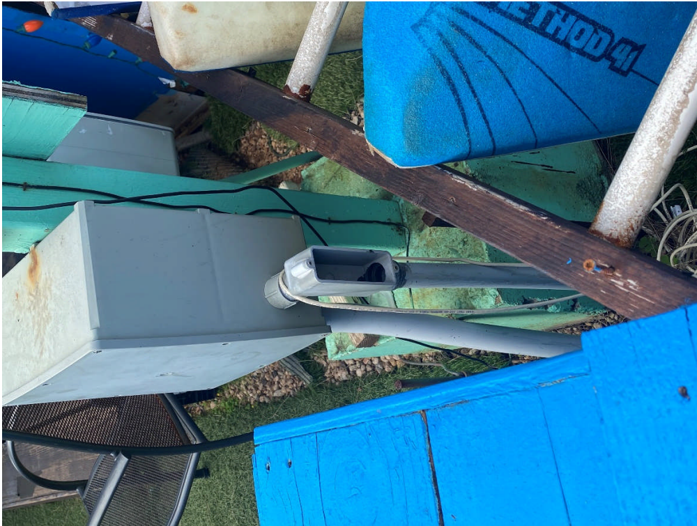
Electrical Code Photo 7
