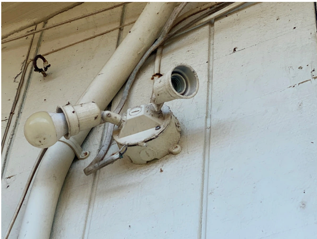
Electrical Code Photo 2
