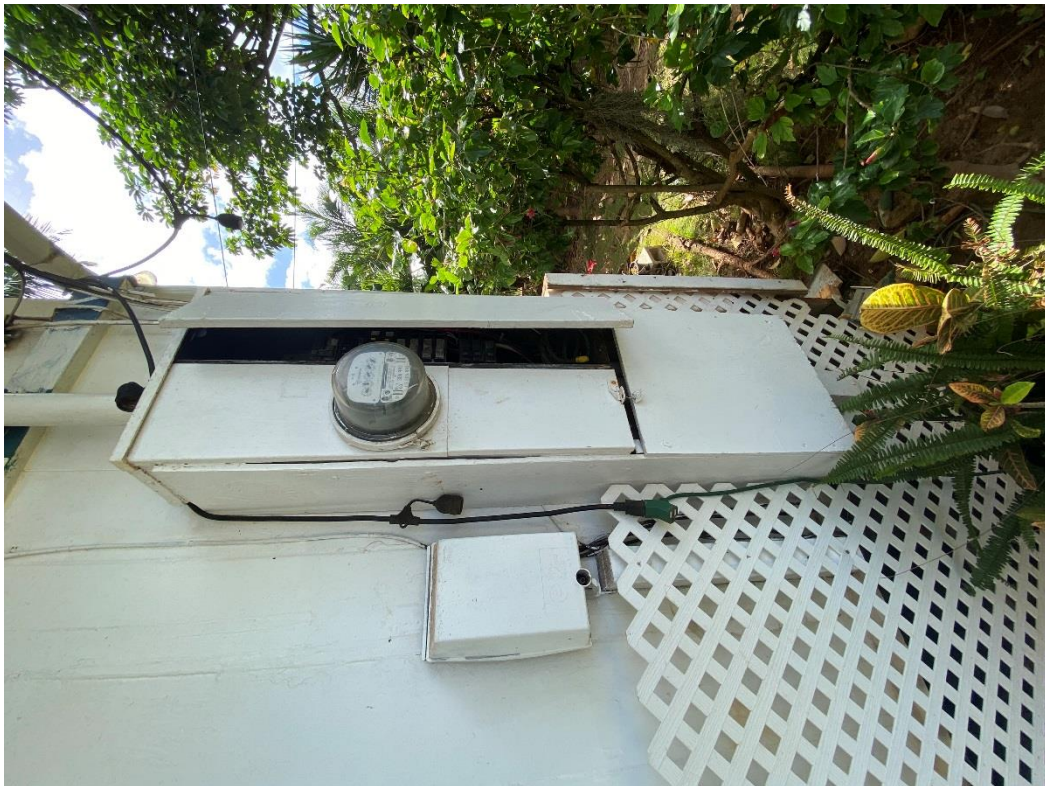
Electrical Code Photo 22
