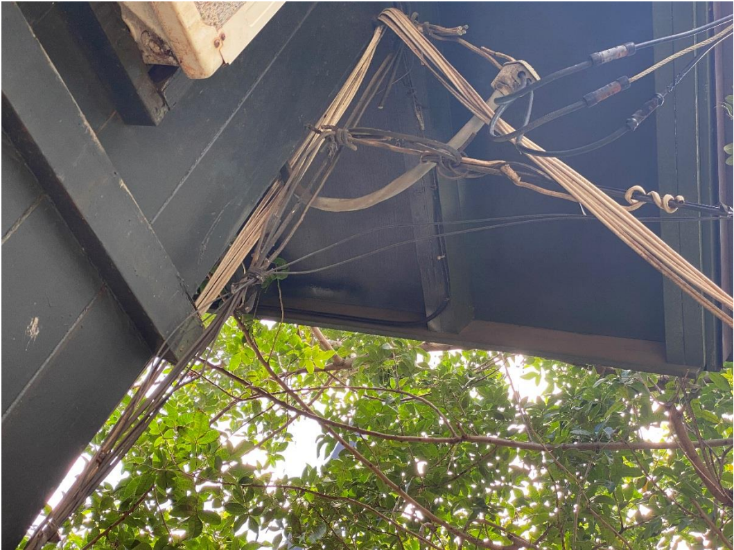
Electrical Code Photo 26
