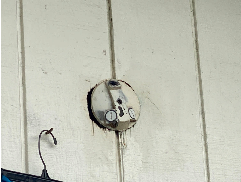
Electrical Code Photo 5
