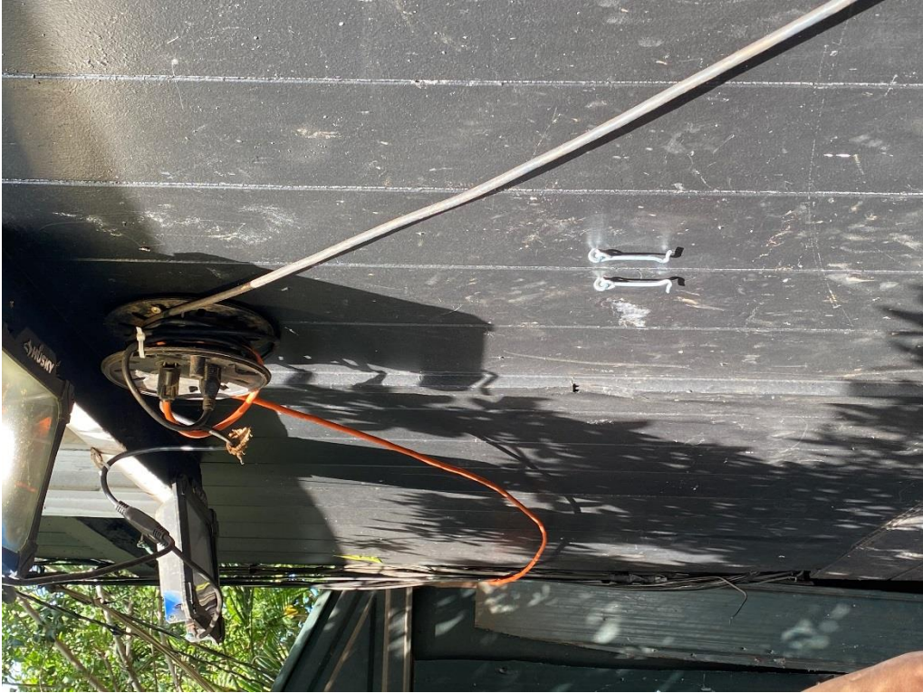
Electrical Code Photo 33
