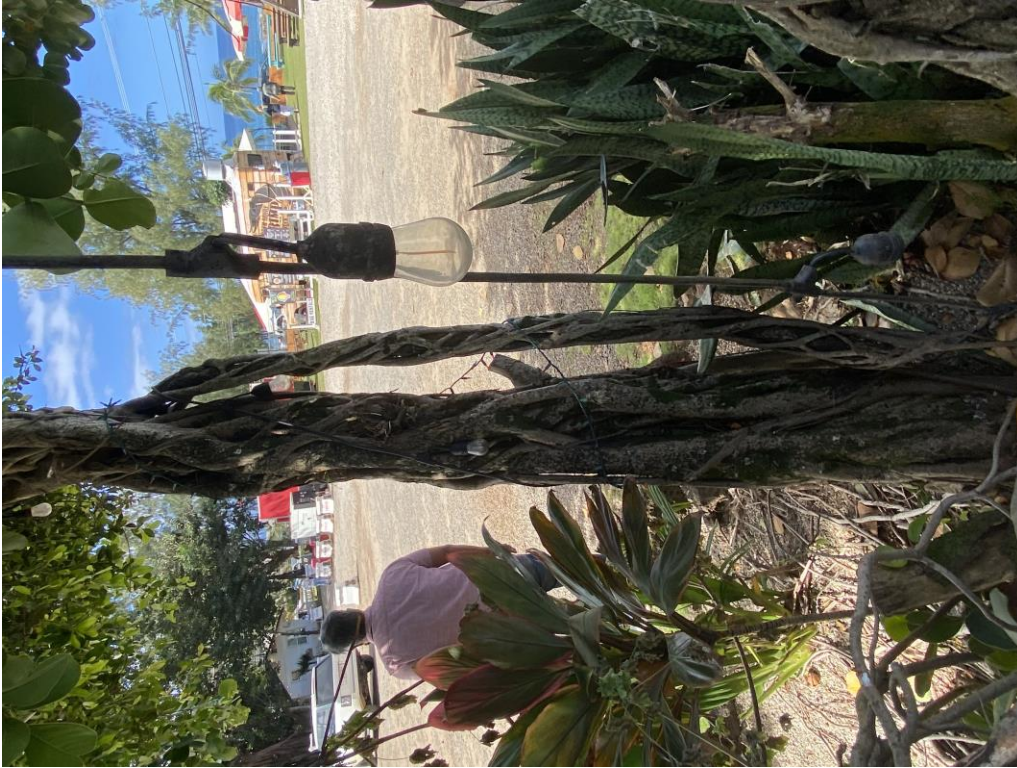
Electrical Code Photo 50
