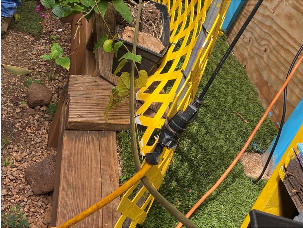
Electrical Code Photo 27
