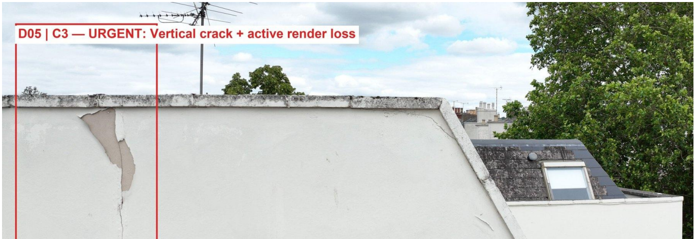
Full-height parapet crack with active render loss, one of four water routes traced (annotated report photo).
