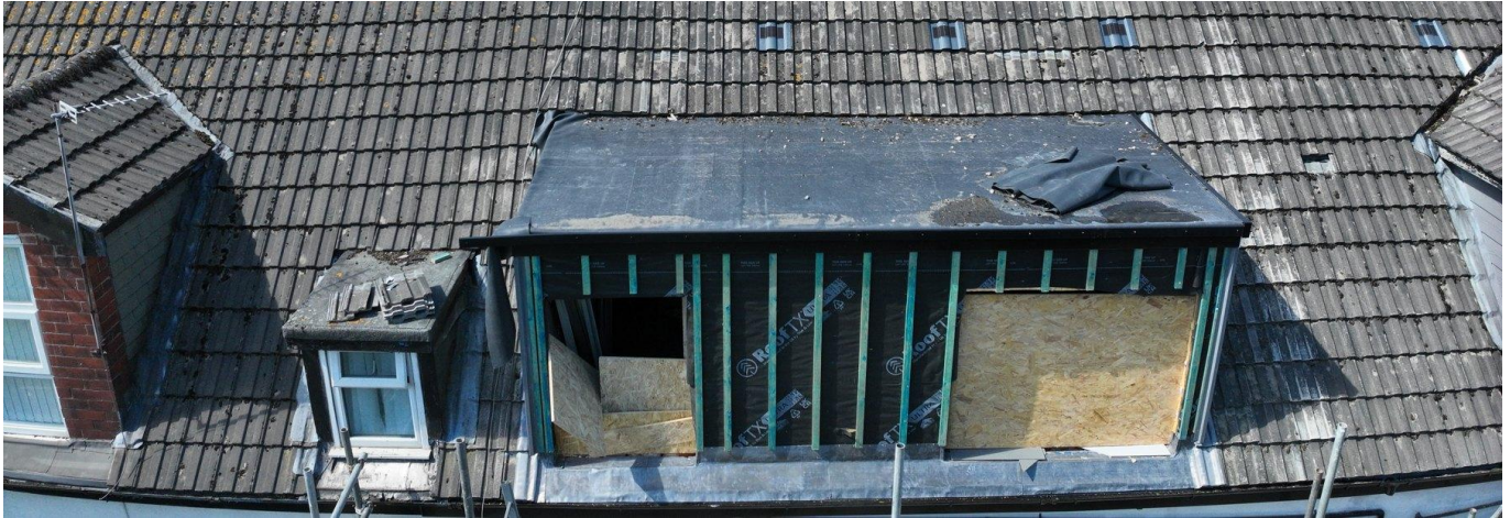
The new box dormer on the day of the check, not yet clad or weathertight (inspection photo, shown with the owner's permission).
