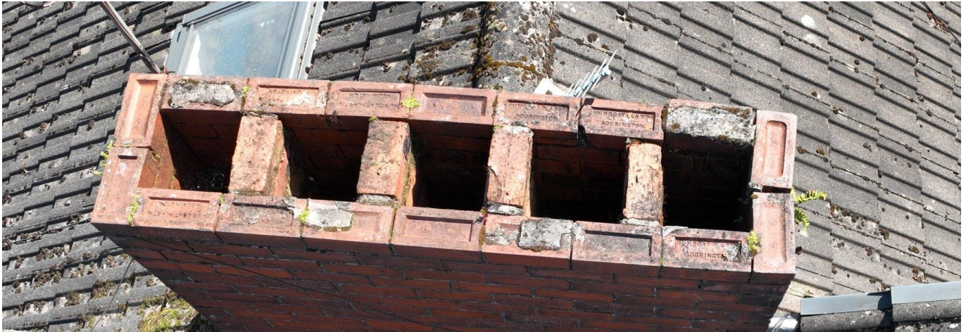
Five open flues with no caps, and plants rooted in the chimney joints. Example survey, shown with the owner's permission.
