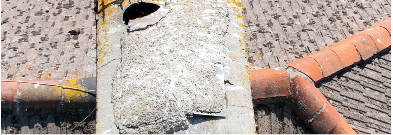
Chimney cap holed, cracked and previously patched: one of three failing systems traced (inspection photo).
