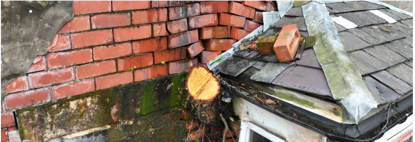
Upper side elevation: missing and displaced brickwork with vegetation growing in the wall (inspection photo).
