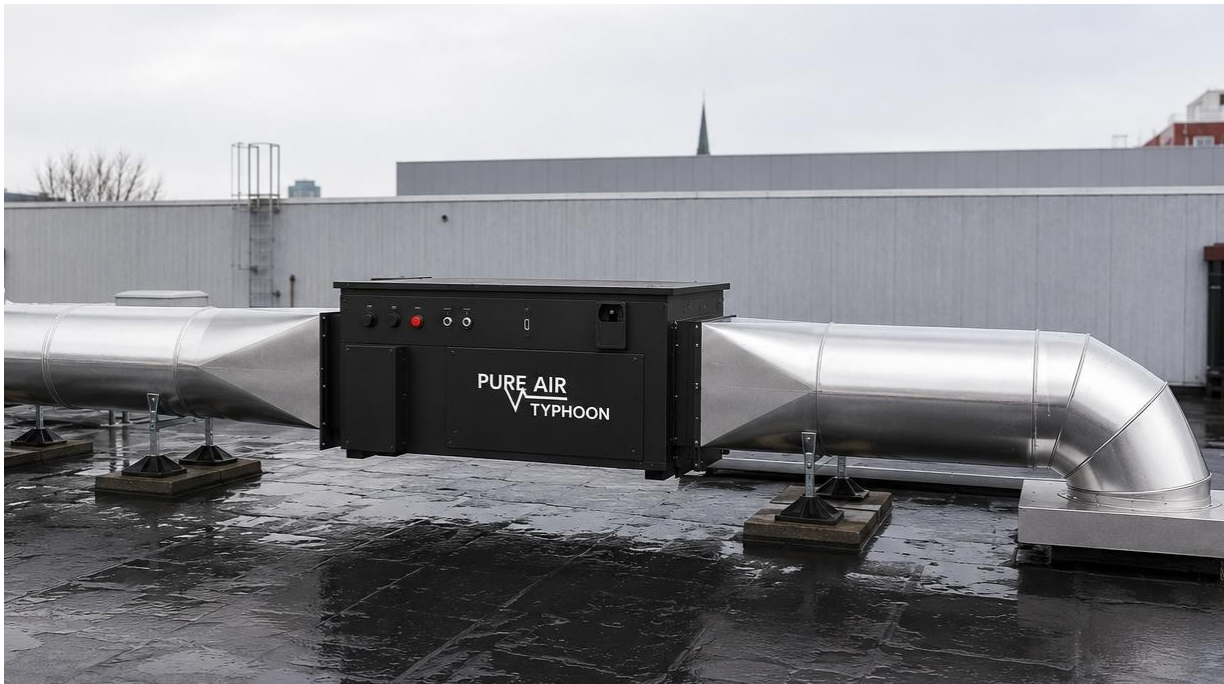
The PureAir Typhoon installed inline into external rooftop ducting run.
