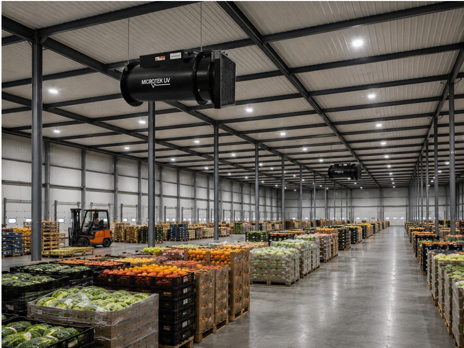
The PureAir Vortex 2 suspended above pallet storage in a distribution warehouse.
