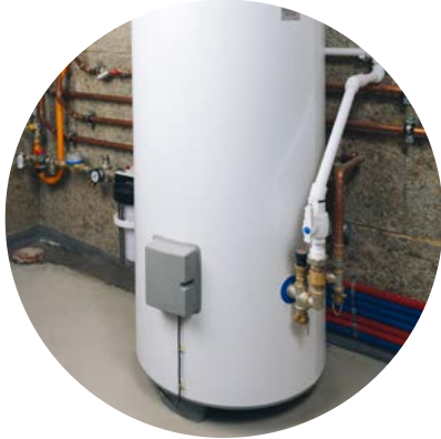
Hot Water units
