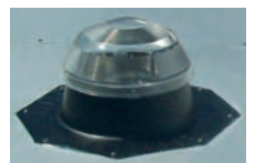
No pitch for over flashing
