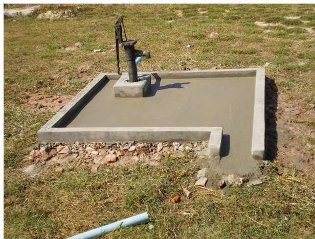
Cast Iron Pump Well
