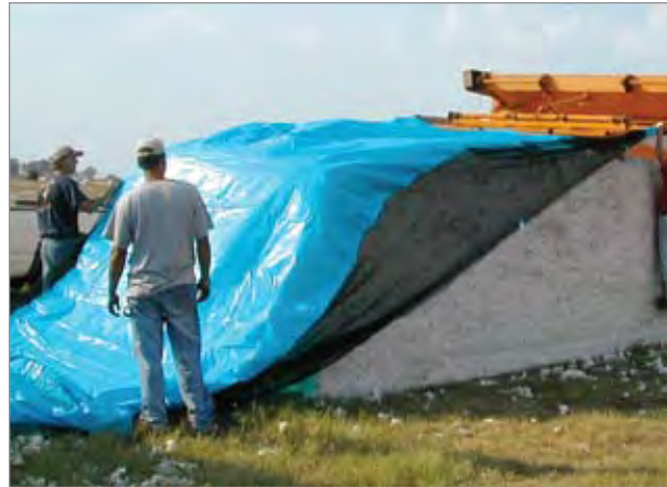
Figure 13 Covering a module by using the builder to pull the cover over the module. The front edge of the cover is attached temporarily to the door as the builder is driven forward.
