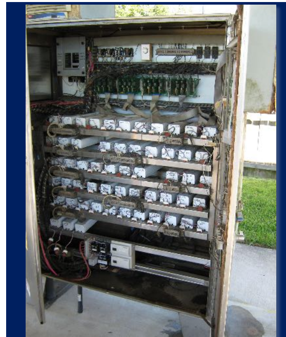
Old magnetic ballasts were inefficient and took up space.
