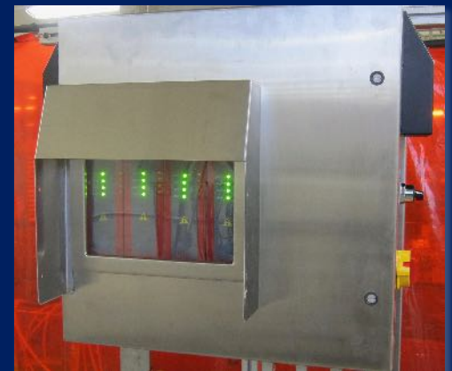
Typical control center. If outdoors, a protective structure helps operation and increases longevity.
