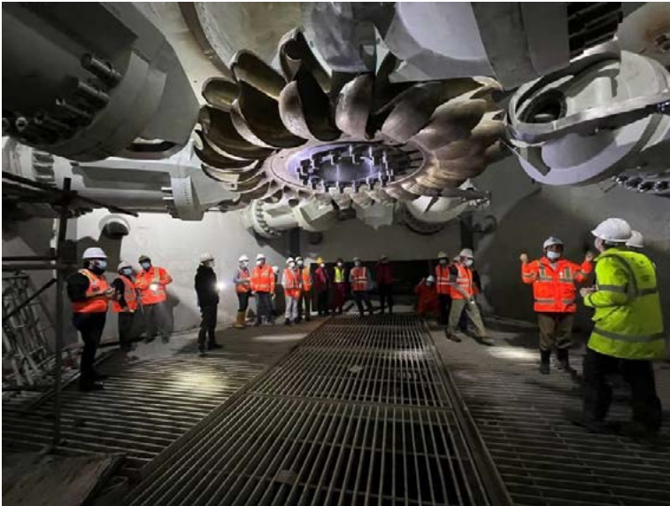
Photo 7 Runner chamber of Pelton turbine
