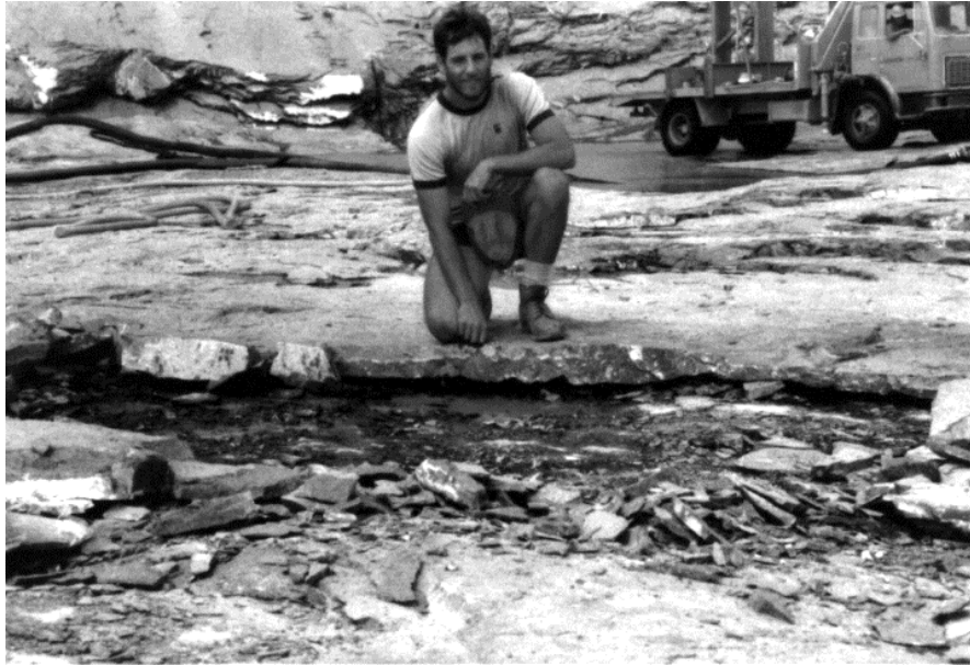
Figure 1 Example of stress relief joint at Burdekin Falls Dam in Fell et al (2015)
