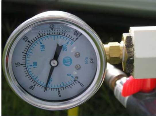
Figure 6 Pressure gauge allowing depth of depression to be set using ball valves (red handle in lower right).
