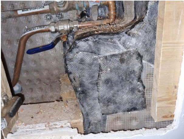
Photograph showing the limited view gained of 'Type C' waterproofing system to basement walls.
