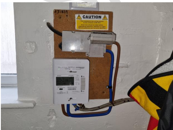
General photograph of electricity meter.
