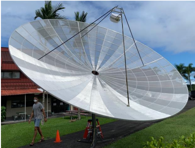
Figure 4. Construction of first 6-meter dish. The receiver is located at the prime focus. Optical fiber and DC power is routed along the lower feed leg.
