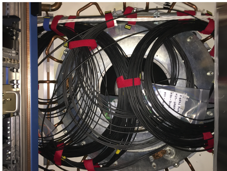
Figure 9 – View of excess fiber cable in Receiver Cabin looking toward the right Elevation Axis.
