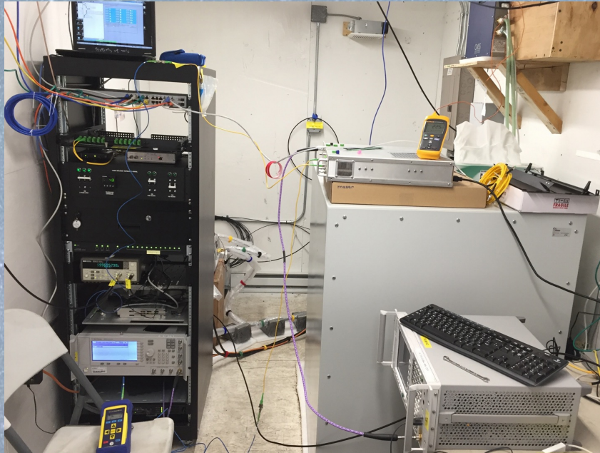
Equipment Rack and Maser Unit
