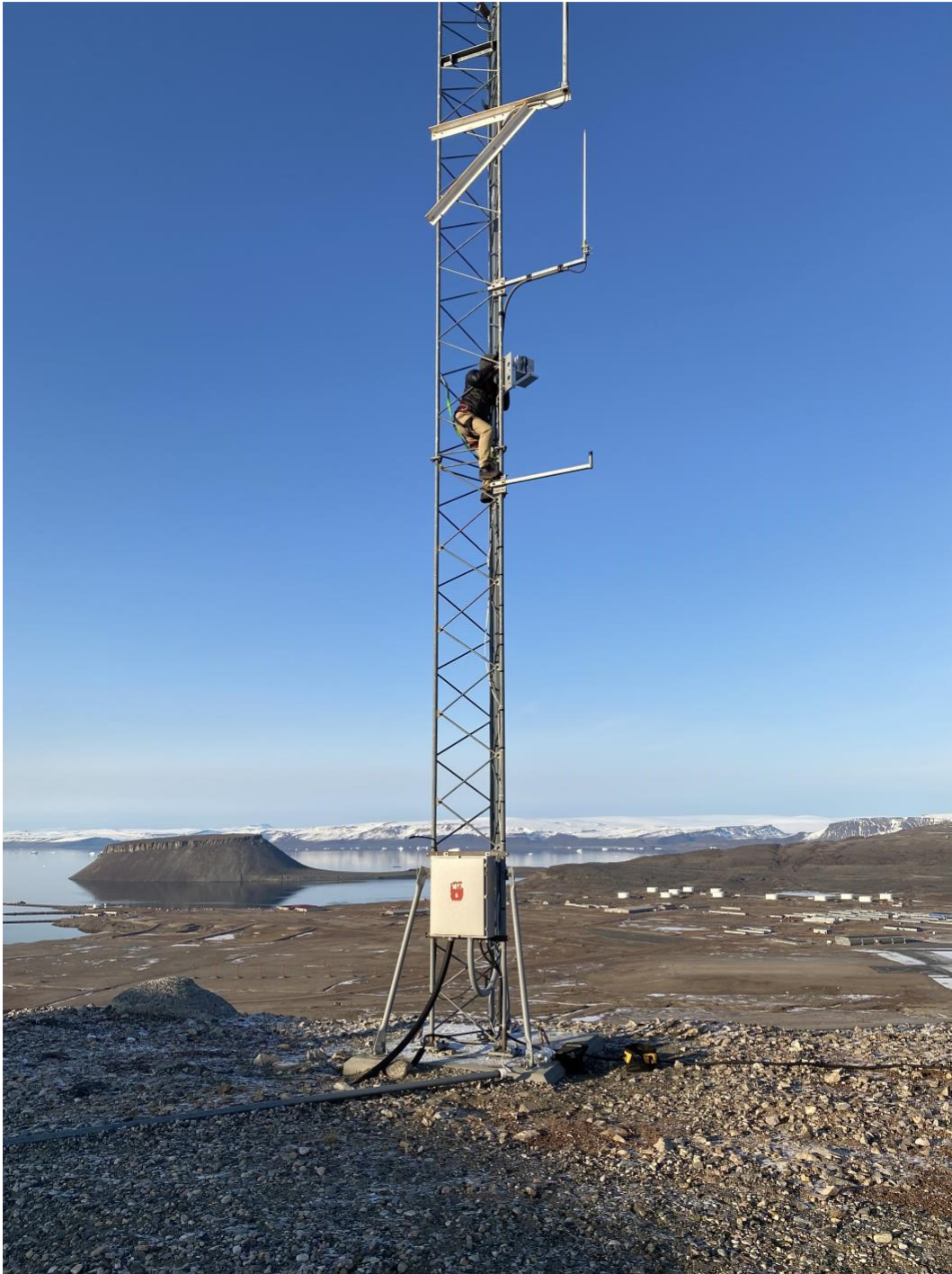
Figure 5. Current transmitter on tower located approximately 3.5 meters above the base. Note the above ground metal conduit carrying the DC power cable from Bldg-1975 located about 30 meters from the tower.
