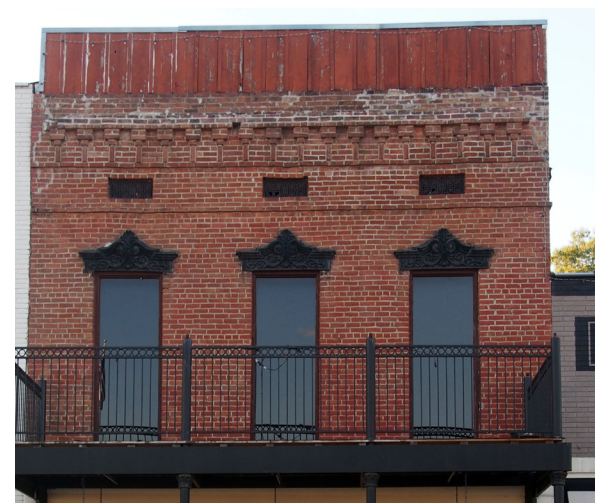
Second story façade with brick corbeling, cast iron window hoods and vents.
