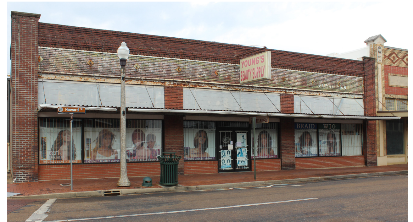
Infilled transoms, storefronts and incompatible entry doors have negatively affected the historic character of this buildings.
