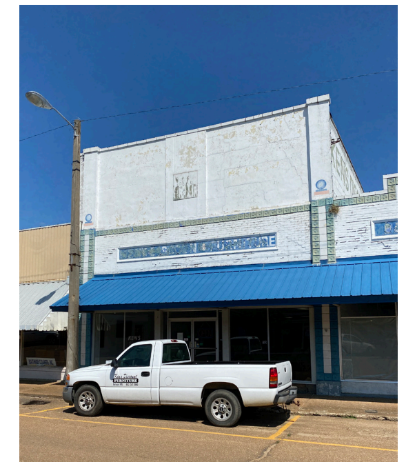
This roof addition has negatively affected the historic character of the original parapet.
