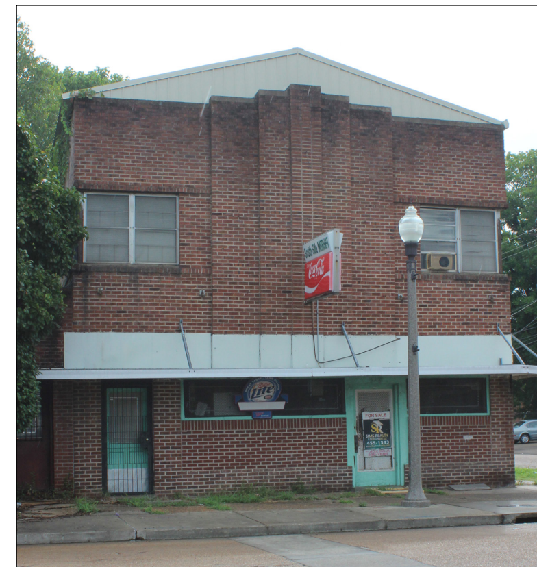
An inappropriate metal gable roof has been added to this brick building.
