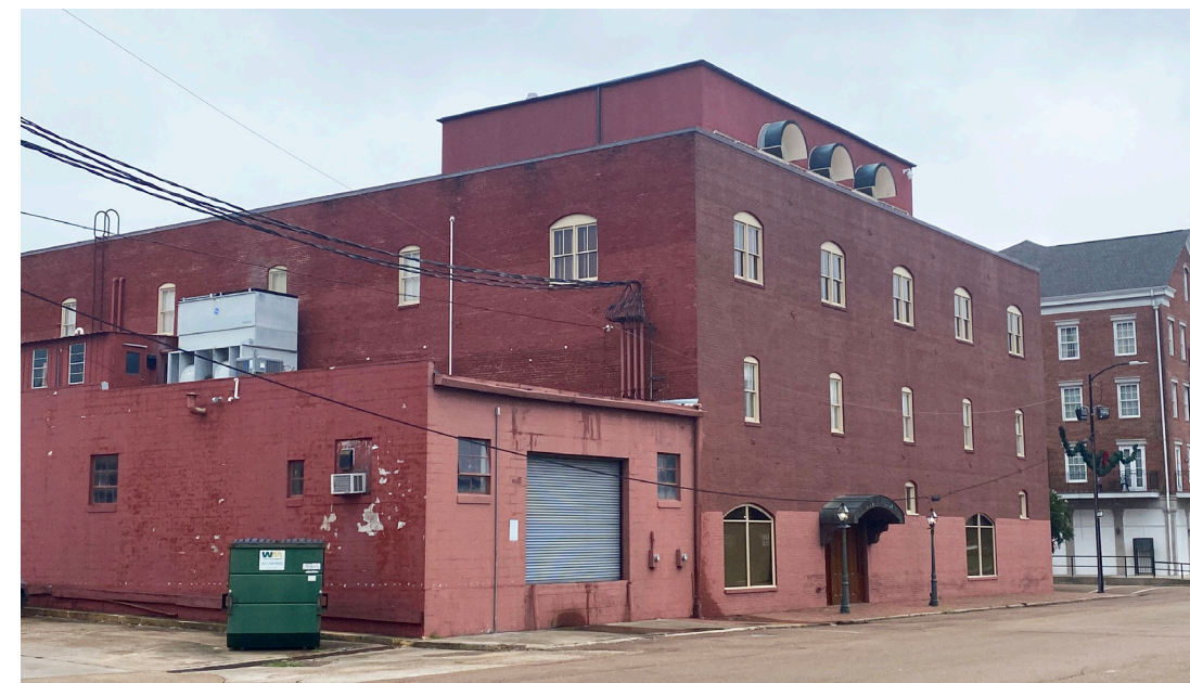
This rooftop addition is only visible from the rear of the building and is unobtrusive in form and color.
