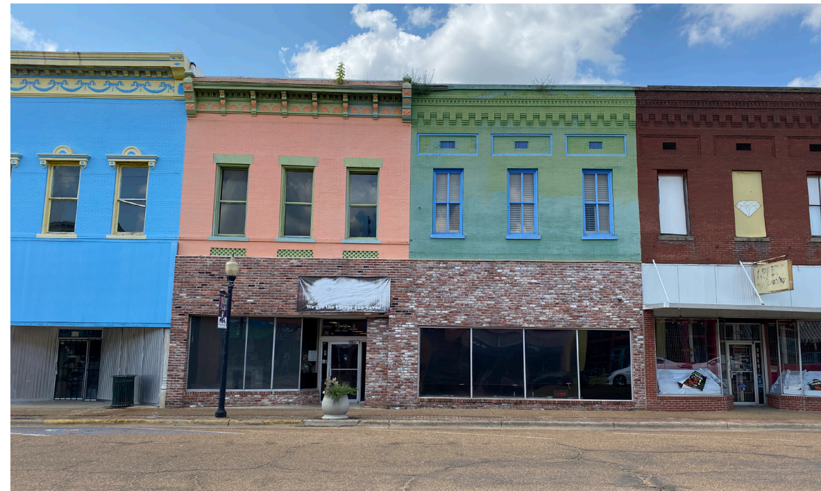
Storefronts negatively altered by the removal or covering of architectural detail and character-defining features.
