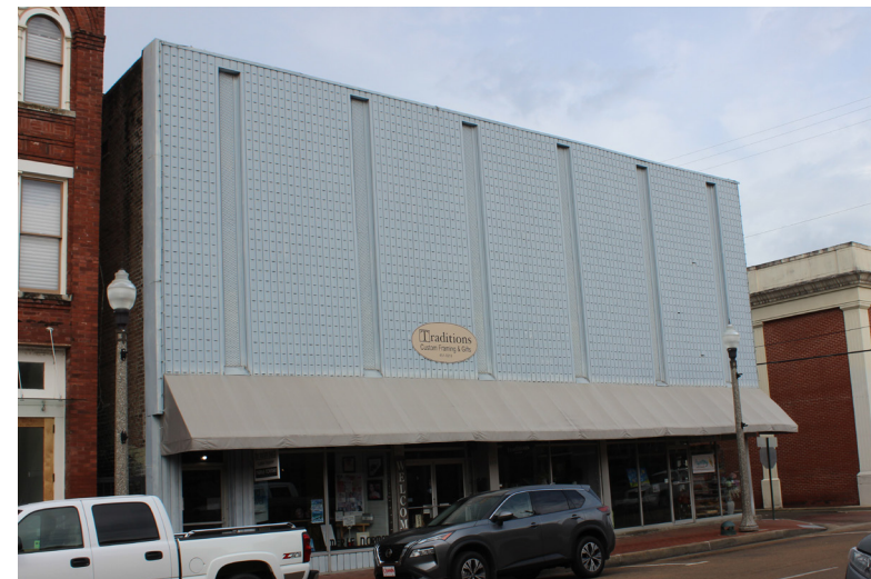
Original façade entirely covered by incompatible metal façade.
