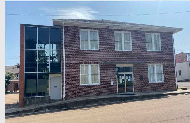
This inappropriate addition is on the main façade of the building and uses incompatible materials, style and form.
