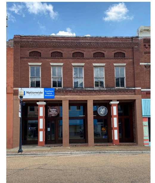
Columns of an inappropriate style have been added to the storefront of this historic building.
