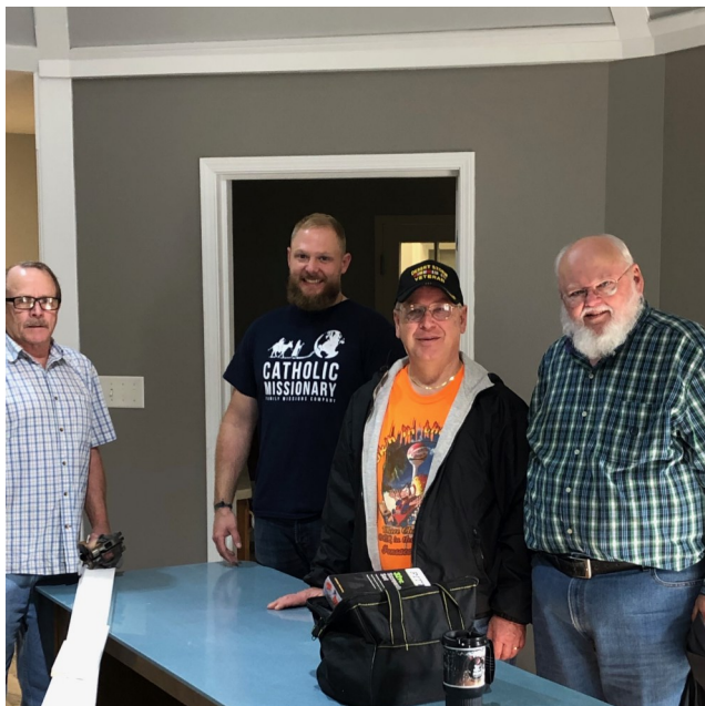
Robert Erisman, Robert Erisman Jr., Dan Arndt, and Ralph Crago help with interior construction at the new Milton Pregnancy Resource Center building.
