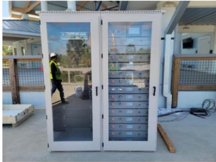
Tampa Electric Site
