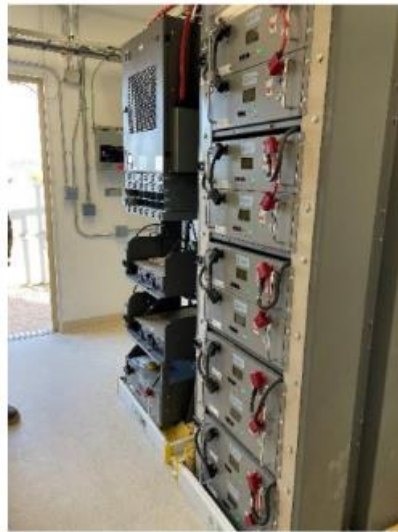
AT&T Cell Site, Alamo, NV
