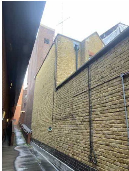
Photograph showing existing separation between the eastern elevation of the M&S building and the houses at nos. 49-51 CIIP. This will be 'filled in' by the new proposal. The header of one of the first-floor windows in no. 51 CIIP is visible in the photograph.
