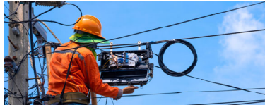
Fiber Communications Network
