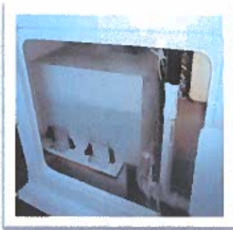
Potable Water Tank
