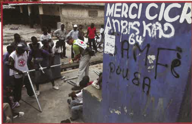
25-01-2010: Port au Prince, Cite soleil. The ICRC sets up a water distribution point with the help of Haitian Red Cross volunteers - M Kokic
