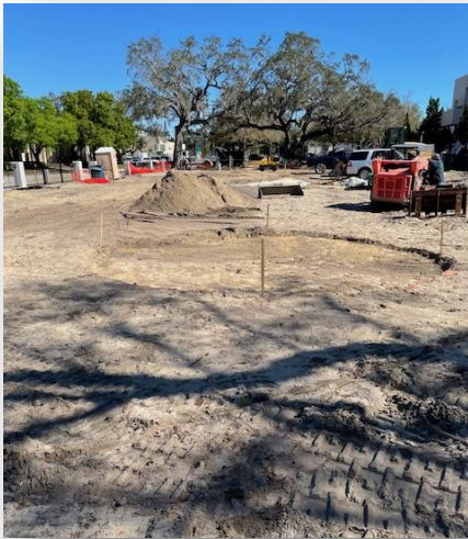
The footer layout for the memorial's circular base at the Commerce Street end of the property.
