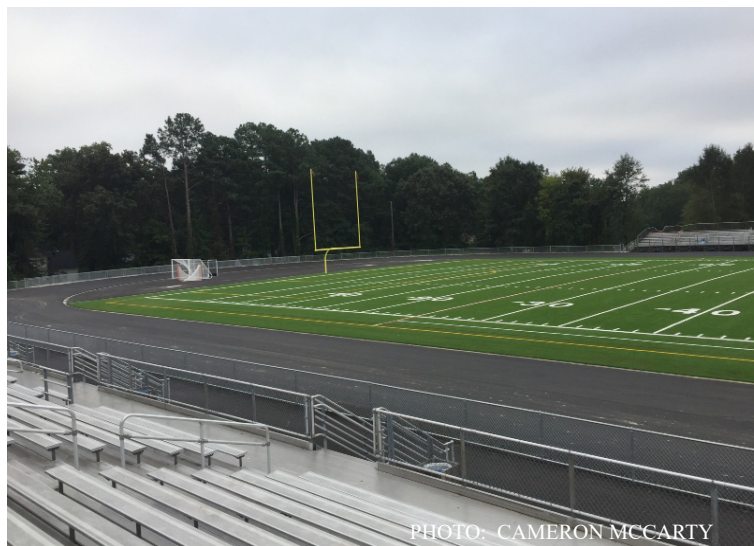
PHOTO: CAMERON MCCARTY The asphalt had to be reconstructed to correct the angle.
