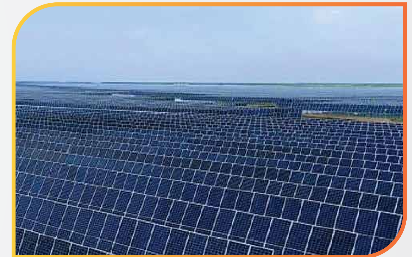
TATA Solar Power Plant 300 MW Operational
