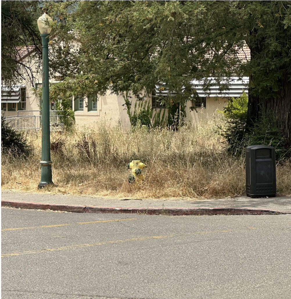
Some fire hydrants on the property have been uncovered but remain out-of-service. (The Sonoma Index-Tribune)
