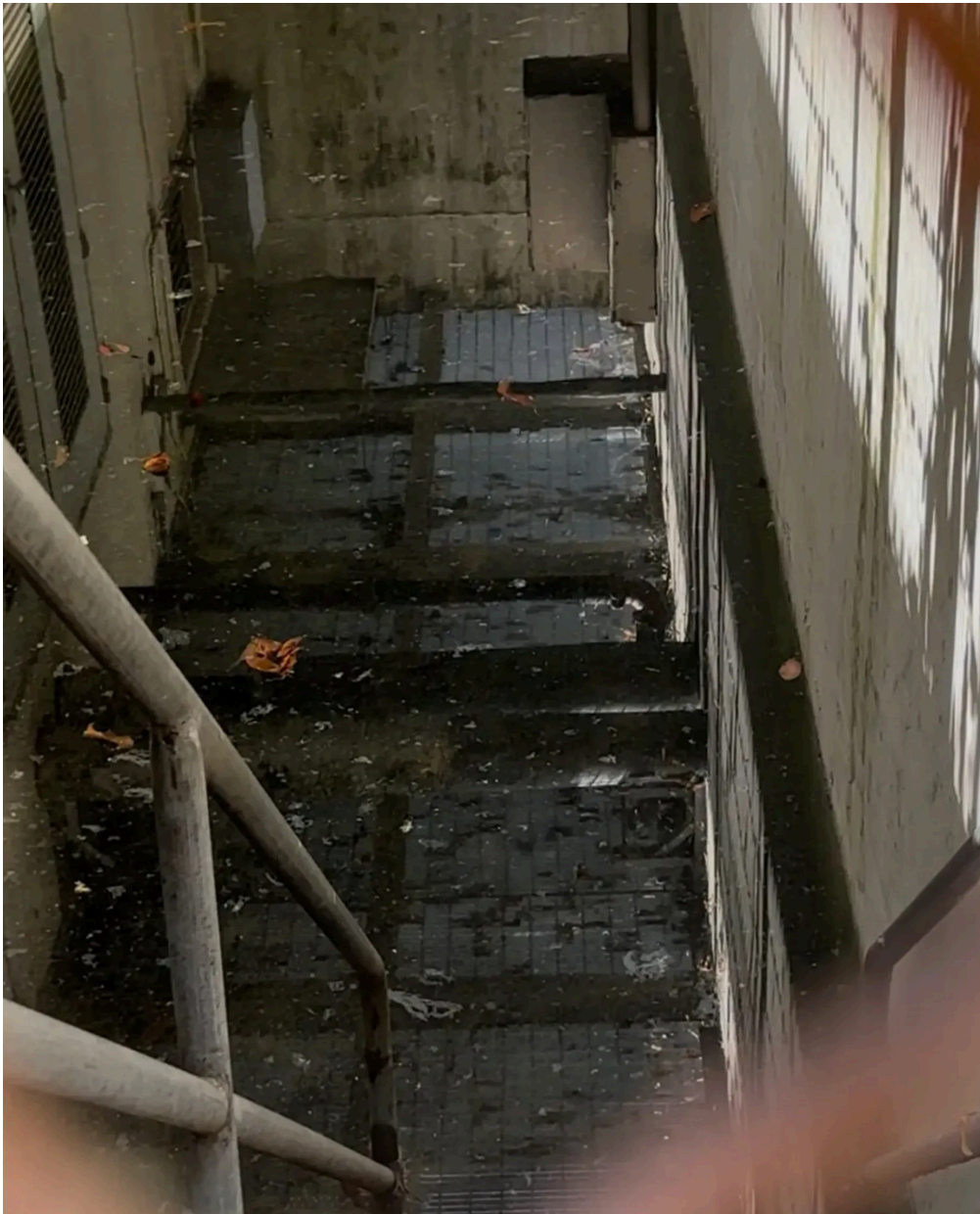
Water accumulates in the basement adjoining the Nelson building on the south end of the Sonoma Developmental Center campus. (The Sonoma Index-Tribune)
