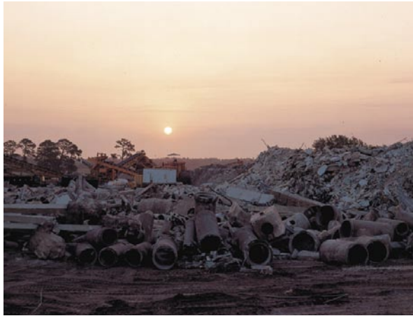
256 buildings, 200 miles of underground utilities, and 25 miles of road were demolished and recycled for the development of Baldwin Park.
