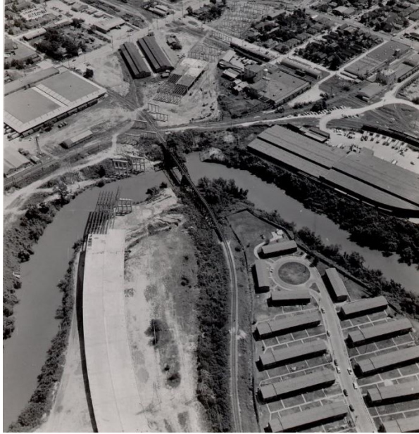
View of highway construction; Clayton Homes public housing development is on the bottom right and Fifth Ward is across the Buffalo Bayou from it (1950s) 220
