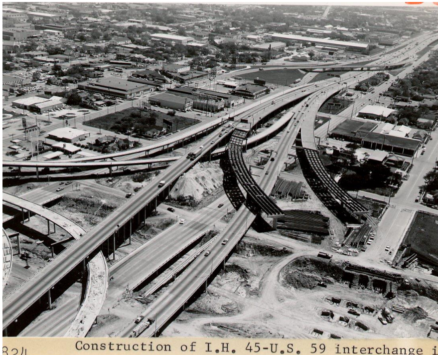
View of construction of I-45 and US-59 Interchange looking southeast and segmenting Third Ward (April 11, 1972) 245
