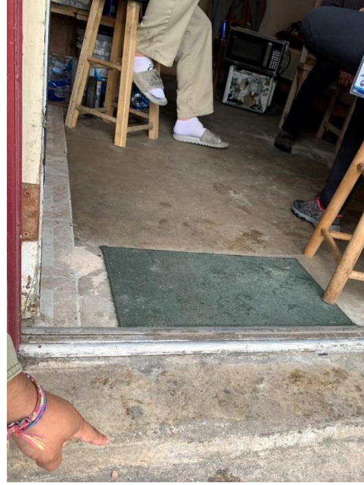
Victoria Manor residents report water reaching the ledge during non-hurricane severe rain events (May 19, 2021)
