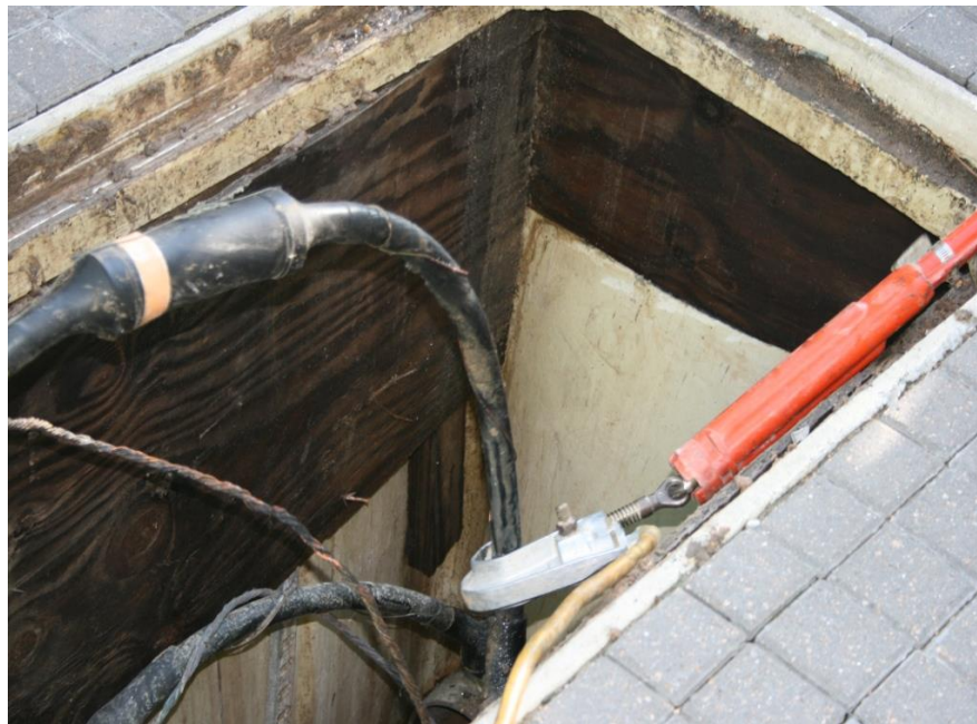
SLIDE 10: Spike Primary cable (Continued)
