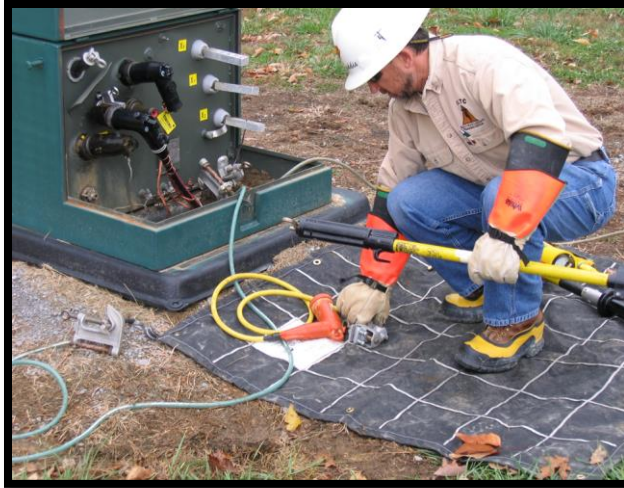
FIGURE 0-1: PAD-MOUNTED TRANSFORMER WORK SITE
