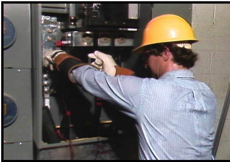
FIGURE O-14: CHECKING SECONDARY VOLTAGE AT THE CUSTOMER'S BREAKER BOX
