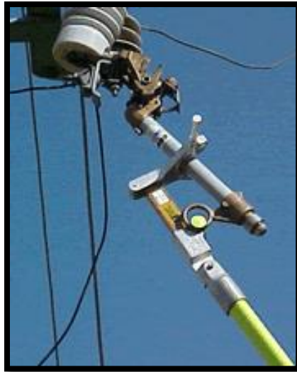
FIGURE 0-12: CLOSING POLE-TOP CUTOUT SWITCHES
