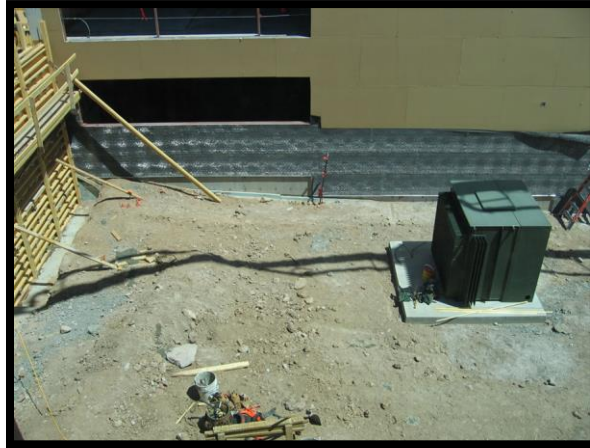
FIGURE 0-3: CONCRETE BASE WITH TRANSFORMER
