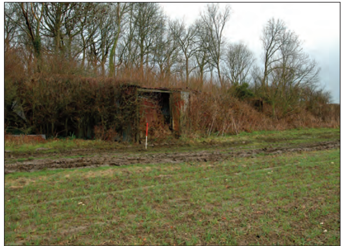
Plate 4 Location of derelict farm building no.1 in Field 2 on the south side of Young Covert, 1m scale
