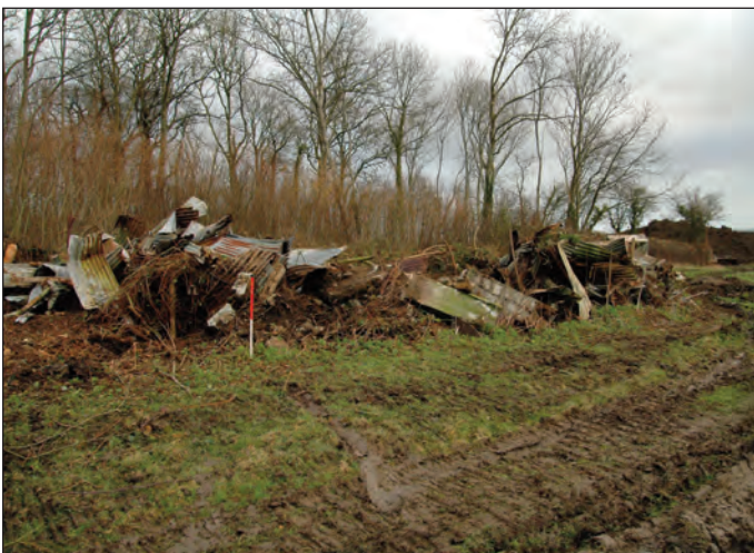
Plate 5 Demolished farm building no.2 on the east side of Field 2, 1m scale
