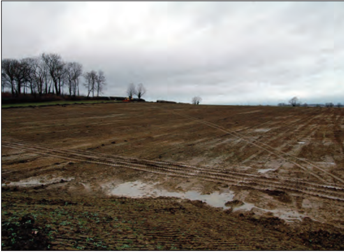
Plate 7 The stripped surface of Field 1, southern end of the excavation area, looking north-west
