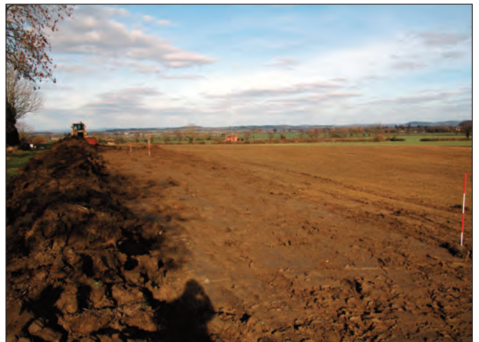
Plate 12 Stripped ploughsoils beside Young Covert on the west side of Field 1, looking north, 2m scale
