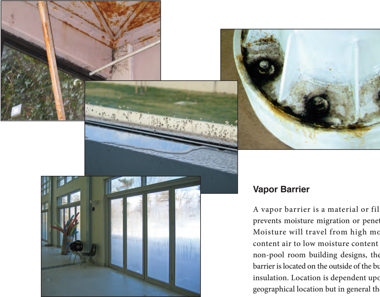
Figure 3. Examples of condensation and poor air distribution.
