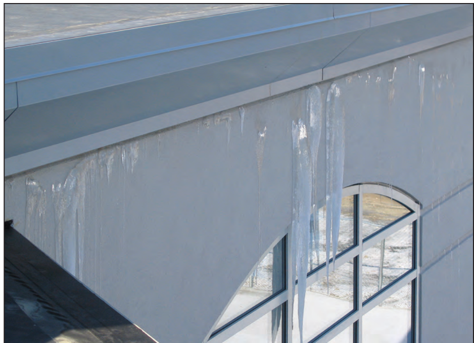
Figure 5. Example of natatorium with improper seals showing moisture migration and icicle formation.
