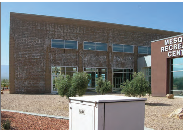
Figure 4. Example of natatorium without vapor barrier showing white chalking on building exterior.
