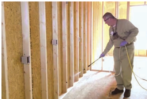
Bora-Care is applied to your homes by your pest company during the dried-in phase of construction.
