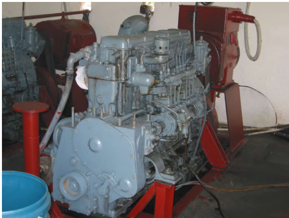
Po Toi Island #8389 Electricity Generator
