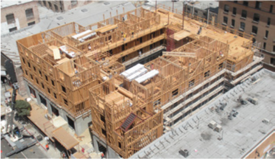
Figure 2.5: A Lightweight timber-frame building under construction in the US – The New Genesis Apartments in Los Angeles, California, designed by Killefer Flammang Architects, is a mixed-use and mixed-income wood-frame building with commercial retail space.
