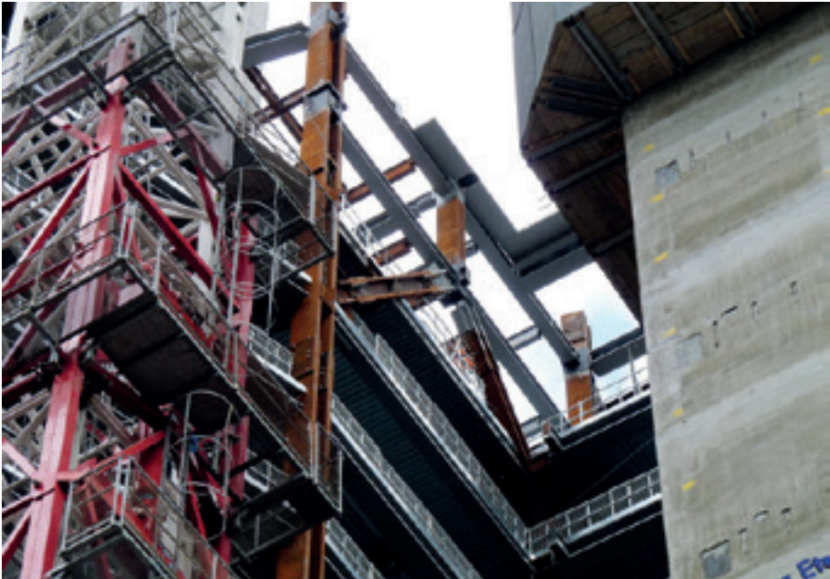
Figure 13.1: Some of the main transfer structures over the backpack/tower interface can be seen above
