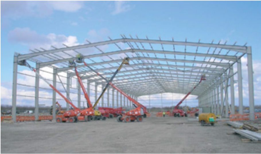
Figure 2.4: A typical steel portal frame shed-style building under construction Photo courtesy of Graham Couchman (SCI)
