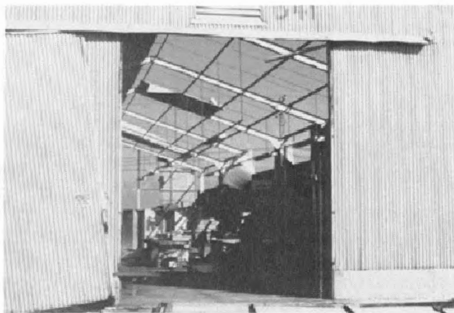
FIGURE 7-17. TYPHOON ALICE DAMAGE, MAINTENANCE SHOP.
