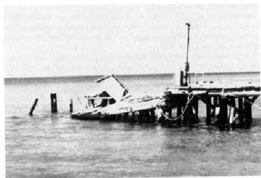
FIGURE 3-2. DELAPIDATED BOAT DOCK.
