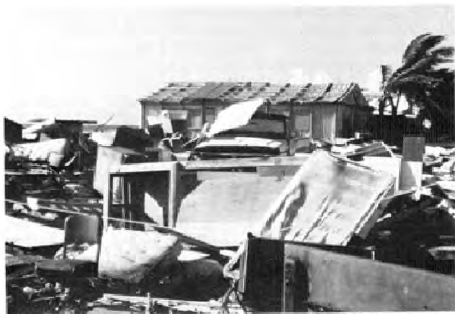
FIGURE 7-16. TYPHOON ALICE DAMAGE, THE "WHITE HOUSE."
